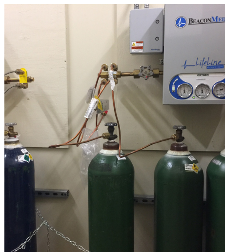
Gas Tank Closet
